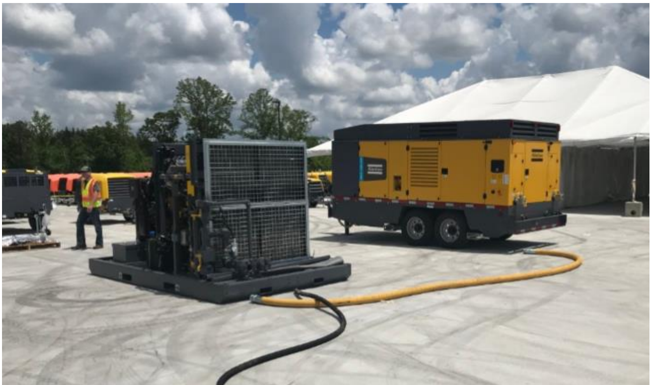
Figure 4 The Atlas Copco booster on the left side of a compressor
