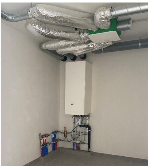
Figure 2 District heating satellite and ventilation system inside apartment
