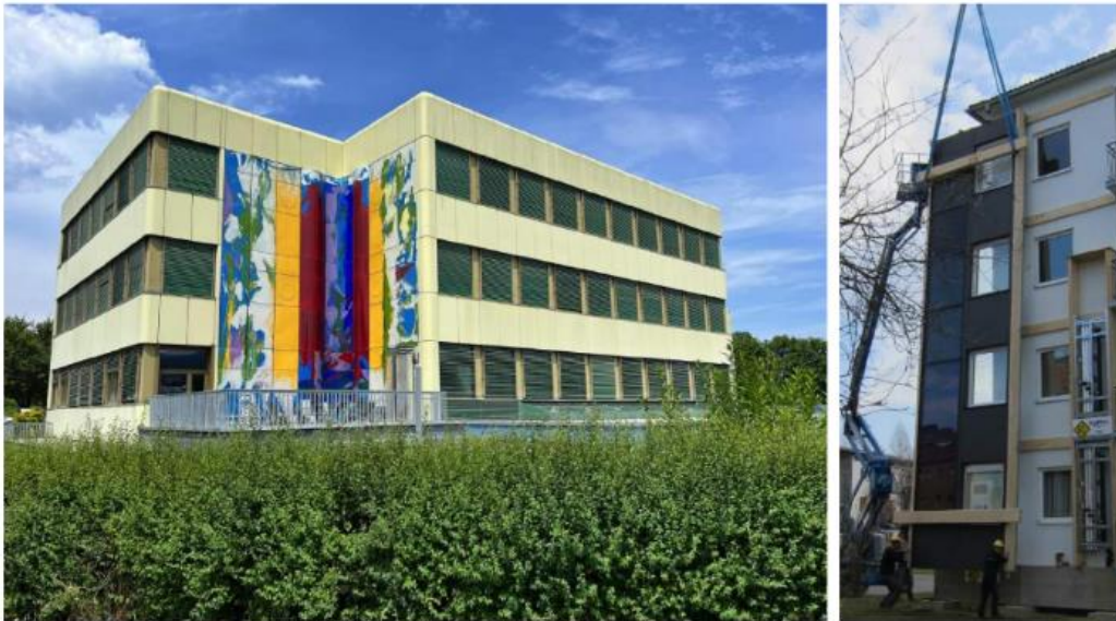
Figure 1: View of the school building in Knittelfeld (left) and impression of a prefabricated facade element being installed (right). Source: Nussmüller Architekten
